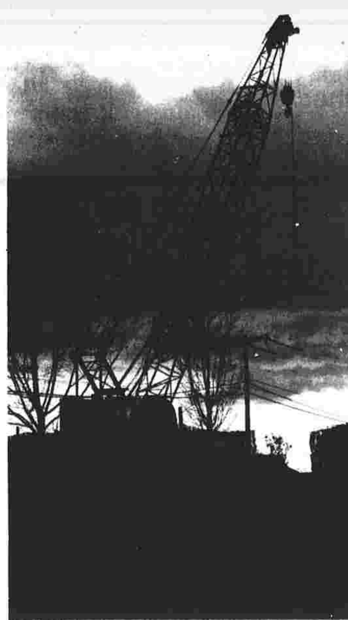
A construction crane, idled by a strike by construction workers throughout the state, stands idle and is silhouetted by the late afternoon sun at the bridge construction project on Demming Street over the Hockanum River. (Herald photo by Burbank)
